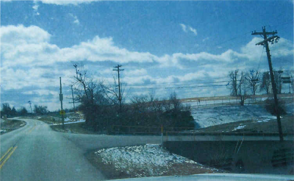
Looking East on KY 1448: rear entrance to Bluegrass Shopping Center (high retaining wall)
